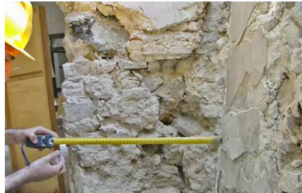
Fig. 2. Chaotic masonry texture made of irregular stone units, poor lime-clay mortar and large inclusions of bricks
